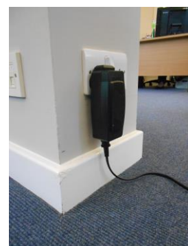
CHARGER PLUGGED DIRECTLY INTO WALL SOCKET
